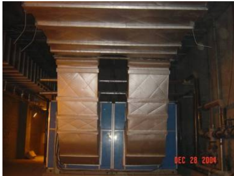
Fig 3.15: Platform Air Handling Unit
