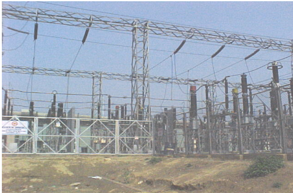
Figure 8.1 : Typical High Voltage Receiving Sub – Station
