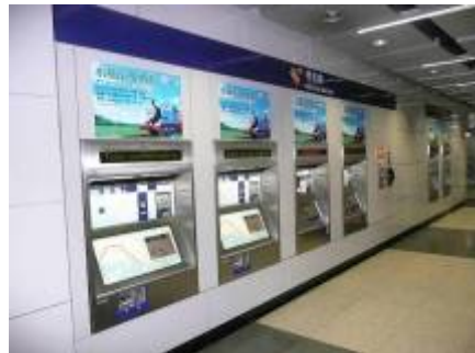
MTR Wall mounted TVM with maintenance corridor in the back – Hong Kong
