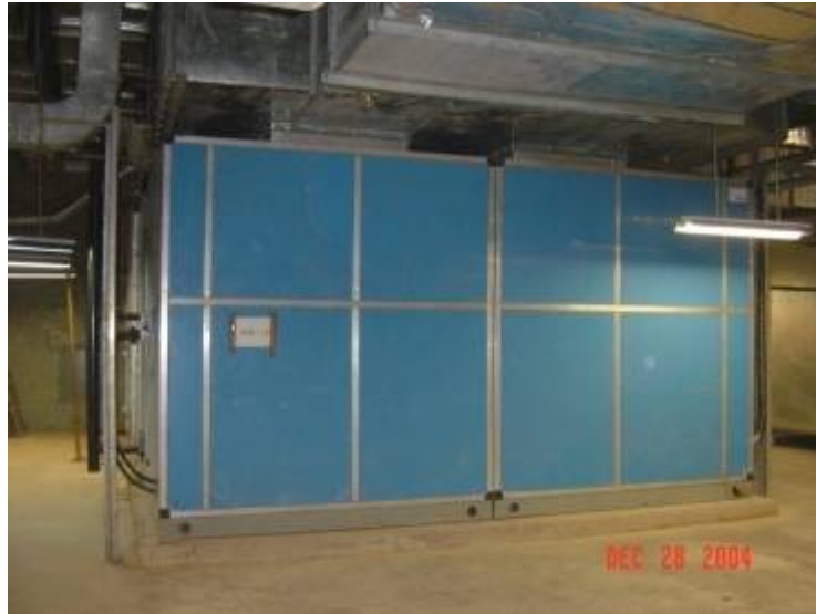
Fig 3.14: Concourse Air Handling Unit
