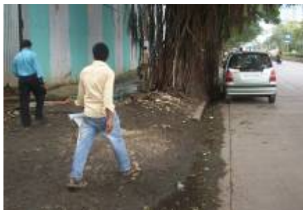
1. Bad condition of footpath creates difficulty for pedestrians
