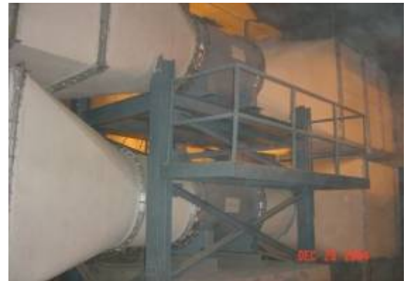
Fig 3.12: Trackway Exhaust Fan
