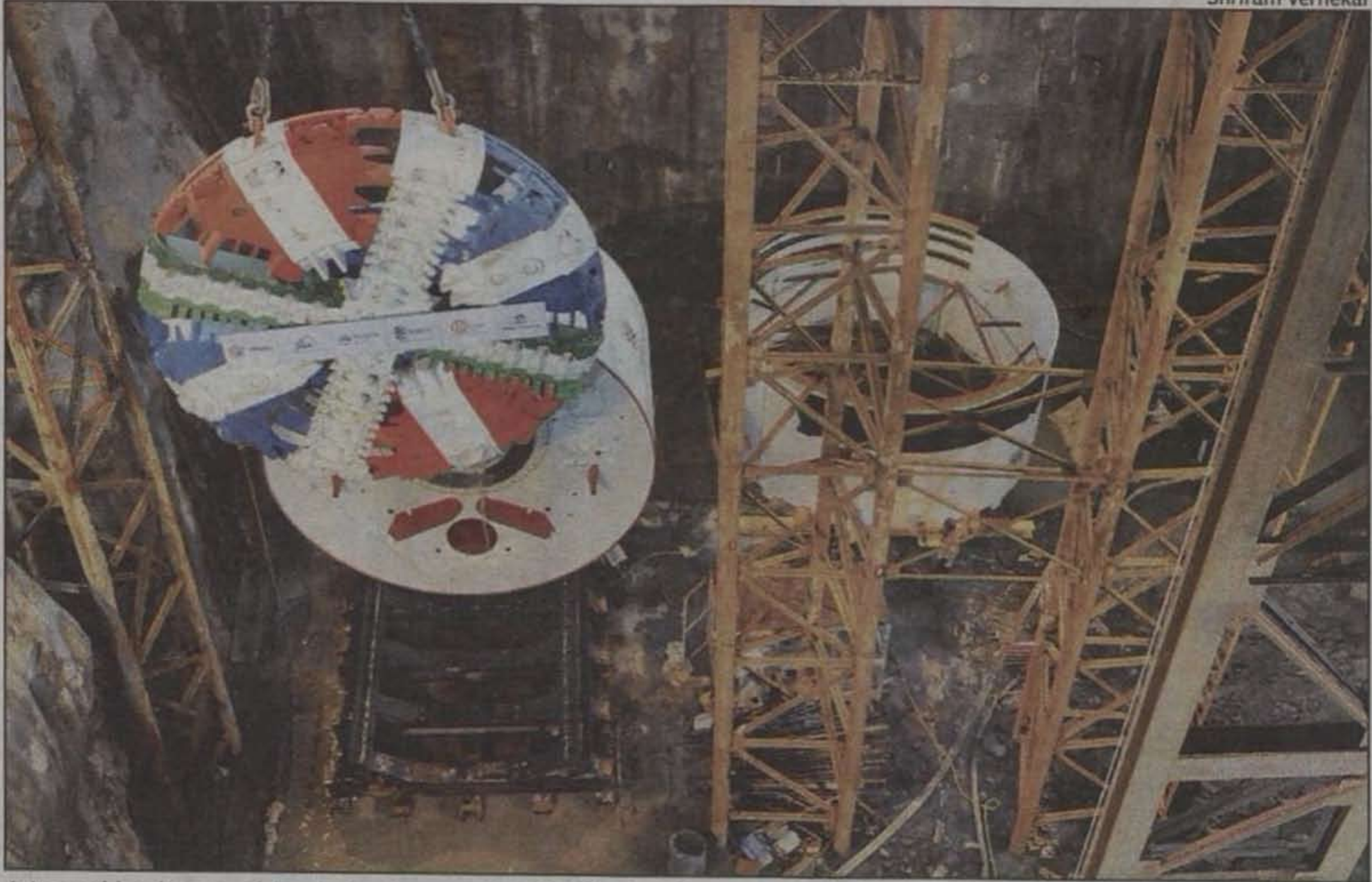
A tunnel boring machine being lowered at Mahim for the Metro II project on Thursday
