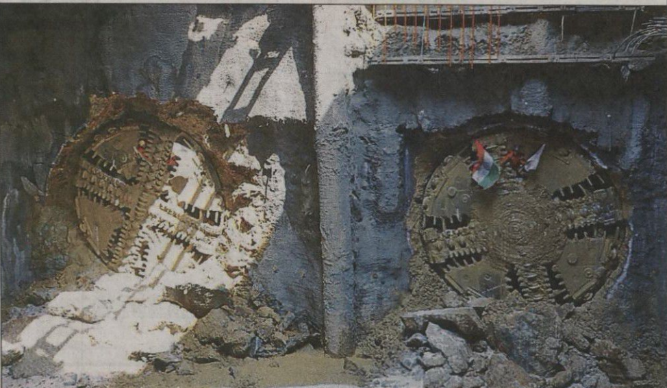
NAYANAGAR-DADAR TUNNEL READY: Krishna 1, lowered on Sept 21 2017, completed 2490 metres of tunnelling on Thursday while Krishna 2, lowered on Oct 18 2017, completed 2472 metres to emerge at Dadar station site
