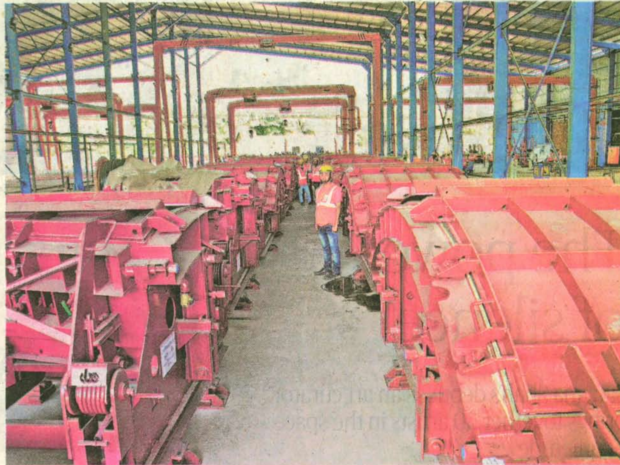
In full swing: The MMRC is fabricating tunnel rings, which will strengthen the underground corridor, at its Wadala casting yard. ■ FILE PHOTO
