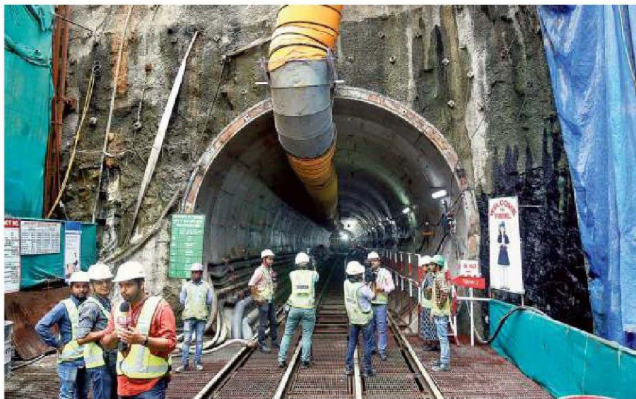
Working hard: MMRCL workers at the tunnel site of the CSMT station of Metro 3. ■ FILE PHOTO
