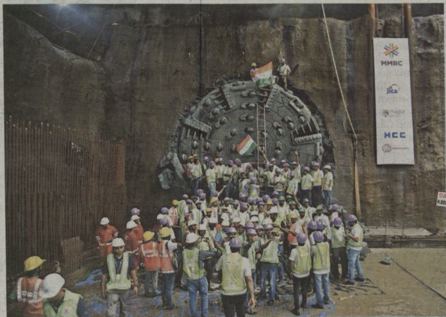
Digging out success: Metro workers celebrate the 15th TBM breakthrough in the Metro 3 corridor on Friday. ■ SPECIAL ARRANGEMENT
