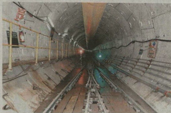
The MMRC has constructed 28 km of the 56 km of tunnels, which will make up 33.5-km line. ■SPECIAL ARRANGEMENT
