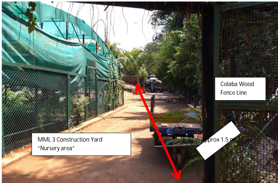
Figure 11 MML 3 Construction area boundary line in Nursery area w.r.t Colaba Wood Garden fence line
