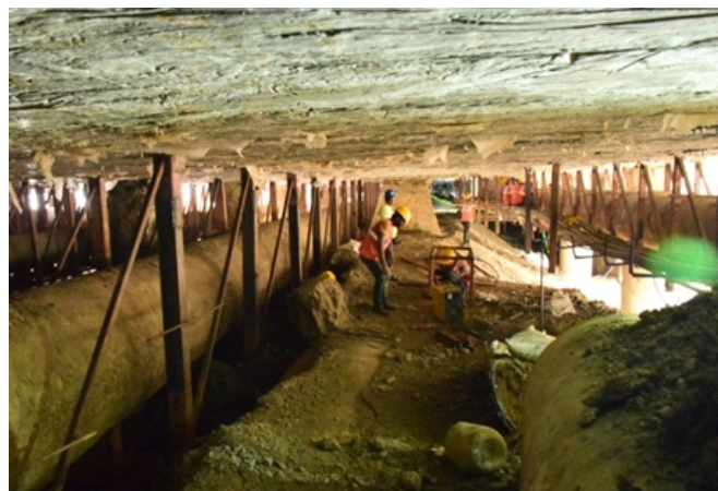
Supporting of existing utilities from traffic decking before taking up station excavation in Acharya Atrre Chowk Station
