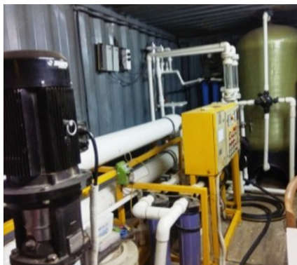
Step 5: RO Plant for advance treatment and reuse for various purposes.
