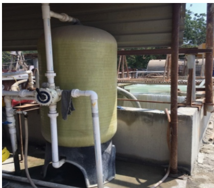
Step 4: Primary treated water is treated with pressure sand filter (tertiary treatment plant)
