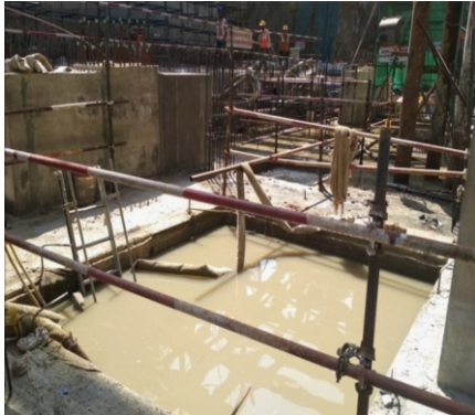
Step 1: Tunnel and station Water collected in sump pits in base slab and retained for suitable time for natural settling of solid particles.
