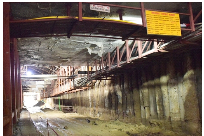
Supporting of water line, Sewer line and power and Telecommunication cables in Acharya Atrre Chowk Station
