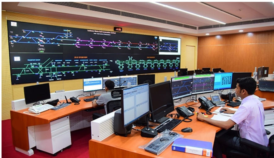
Operations Control Centre (OCC)
