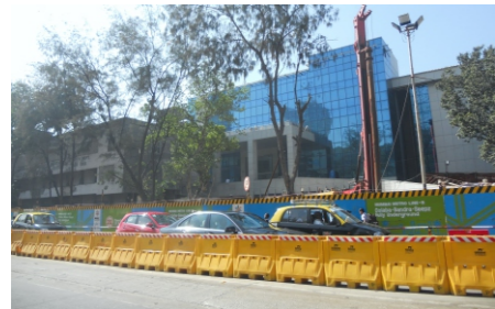
MCGM Engineering Hub
