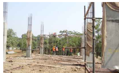
Auxiliary Sub-station Building
