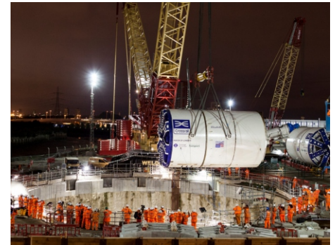
TBM Elizabeth being lowered into launching shaft for London Crossrail (2012) Image Source: www.tunnellingjournal.com
