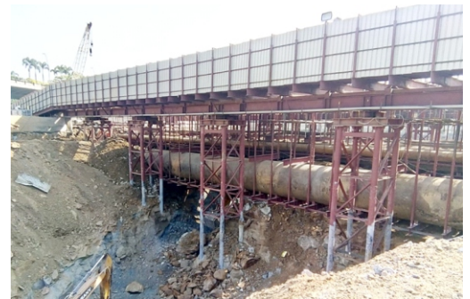
Water mains at Sahar Road Station
