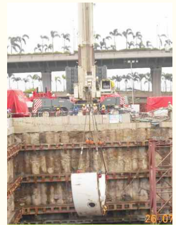
Four TBMs have been lowered at their respective launching shafts and are getting assembled for tunneling.
