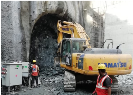
Tunneling by New Austrian Tunneling Method (NATM) commenced at the south end of BKC Station for the 153 m long tunnel below Mithi River. This will facilitate stabling of spare train during operations. This will also act as a Sick Siding.
