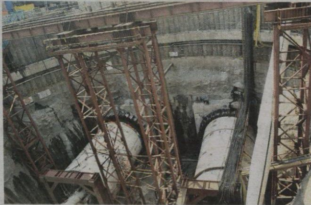
At Naya Nagar in Mahim, TBMs are being used to construct a 33.5-km-long twin tunnel. PICS/DATTA KUMBHAR
