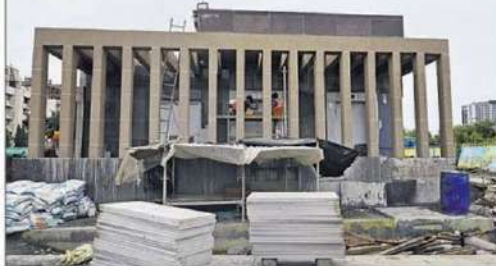
Work going on last month on Phase 1 of the Metro Aqua Line-Aarey-BKC stretch, which is expected to be opened in September. PIC/ASHISH RAJE
