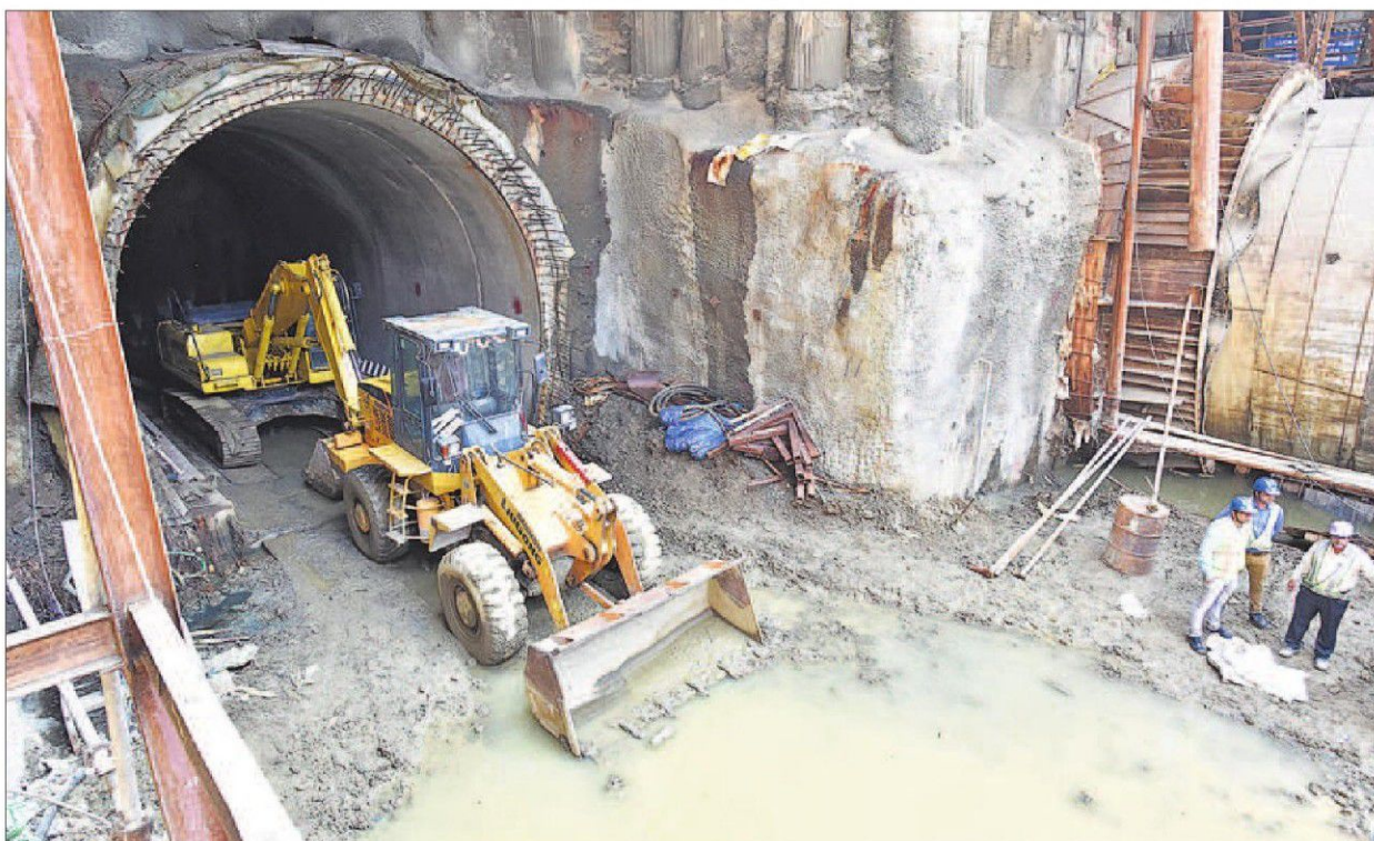
■ Ongoing work for BKC station on Metro-3 corridor below Mithi River at Bandra-Kurla Complex station on Thursday. PHOTOS: ANSHUMAN POYREKAR/HT
