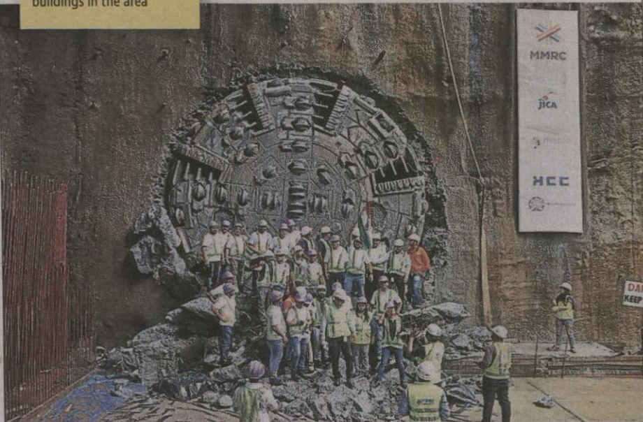
■ MMRC workers at the Mumbai Central station spot after the TBM breakthrough.
