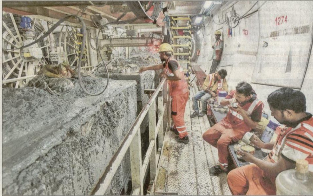
▪ Amid the grime, life down under has to offer some comfort. It comes in the form of an air-conditioned cubicle for workers to have lunch.
