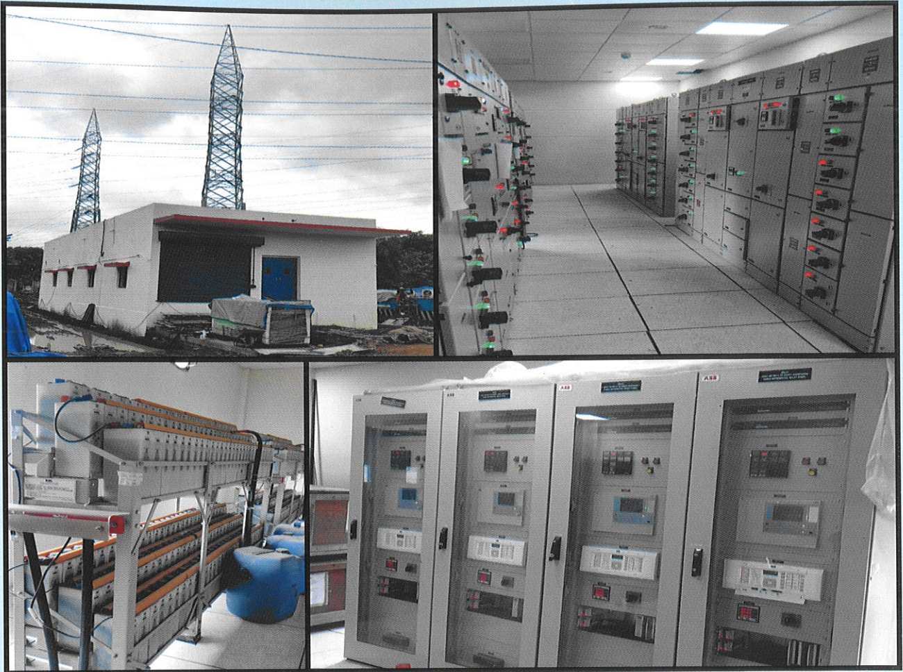
Pylons Termination Yard @ Aarey
