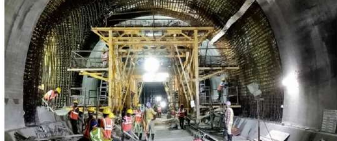
MMRC designed the construction methodology keeping in mind the possible impact on neighbouring buildings.
