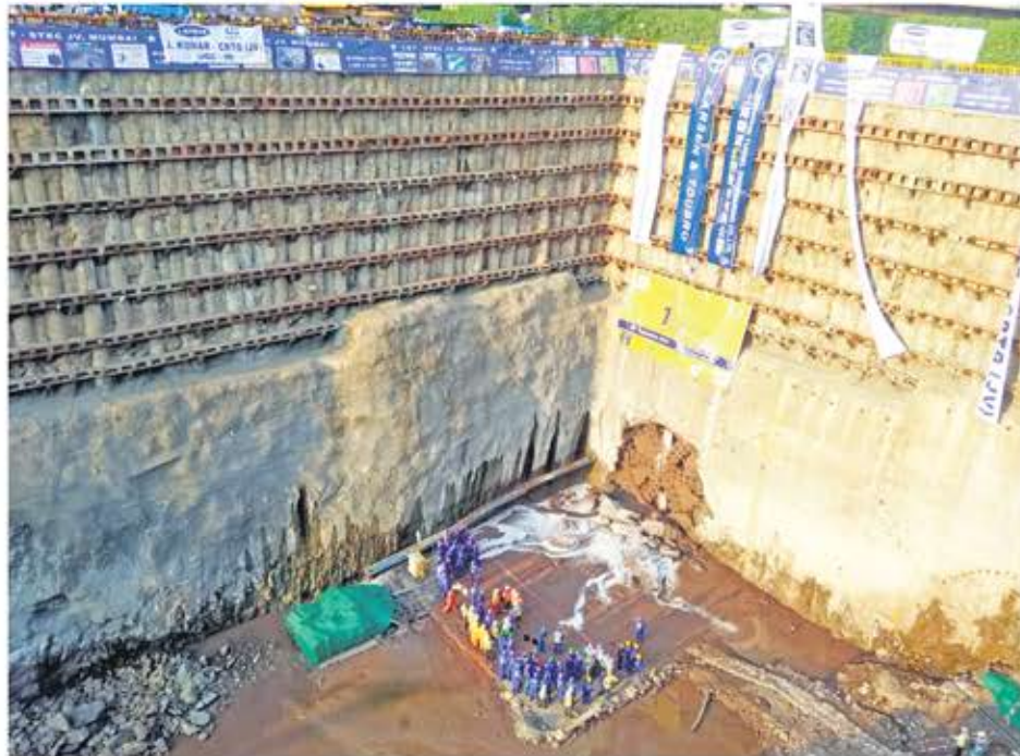
LIGHT AT THE END OF THE TUNNEL: Engineers and workers rejoice as the TBM sees the light of the day after successfully completing boring an underground tunnel for 259 days
